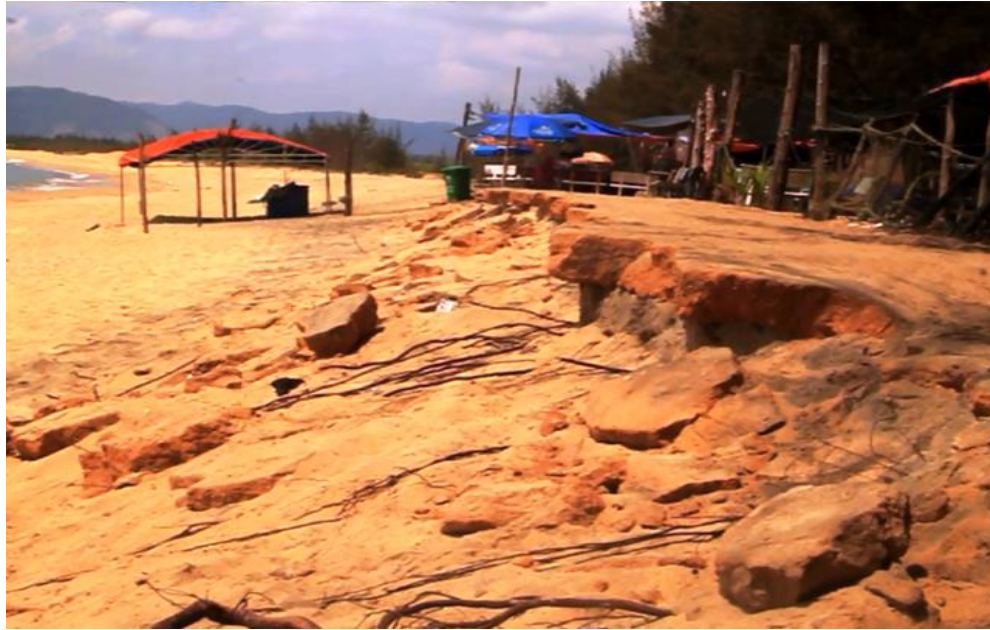
Figure 12. Serious Coastal Erosion in An Quang Đông Village, Phu Cat District, Binh Dinh Province
